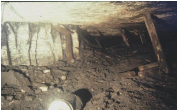
Figure 9. Extrusion of a soft and weak floor material from under a pillar, causing open vertical cracks to develop through the full width of the pillar because of induced lateral tension.
