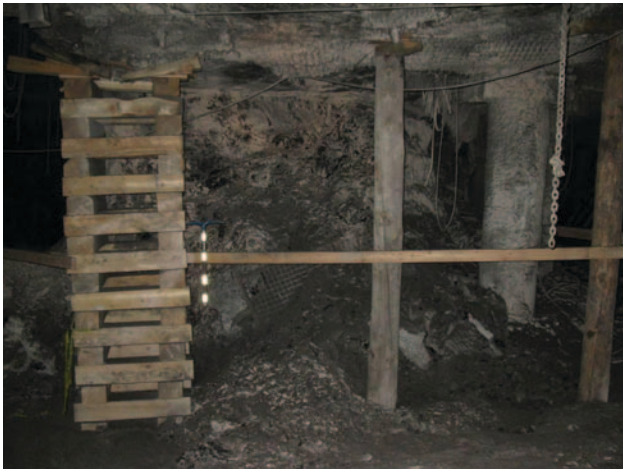
Figure 14. Condition of failed pillar FP-1 at the case study mine.
