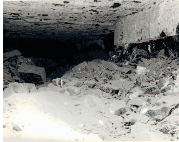
Figure 6. Pillar failure influenced by partings within the seam.
