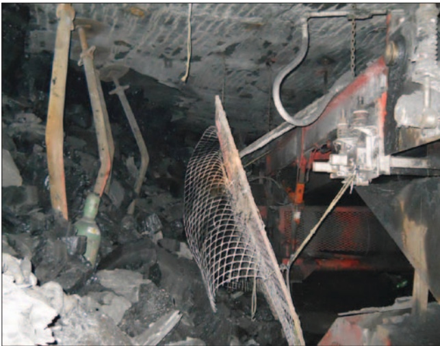
Figure 4. Floor heaving and rib roll has completely covered a belt drive located above the Dorothy barrier pillar.
