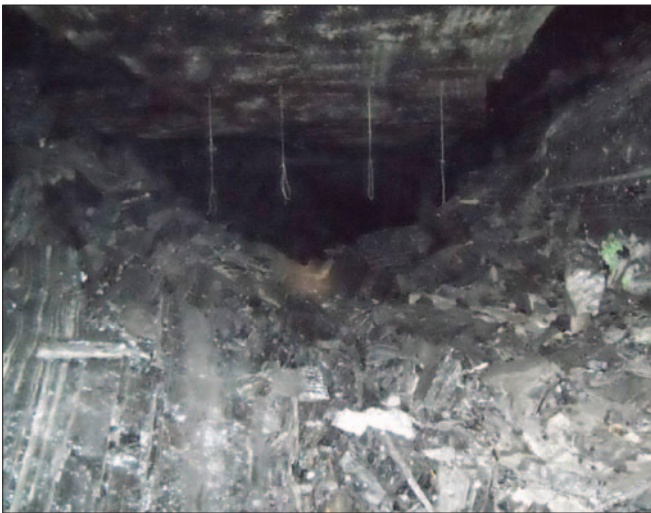
Figure 5. Coalburg entry above the Dorothy barrier pillar almost filled with broken coal, leaving only a 14-ft-wide by 6-ft-high triangular opening.
