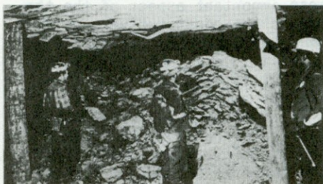
FIG. 2. Floor Heave in Conventional Room.
