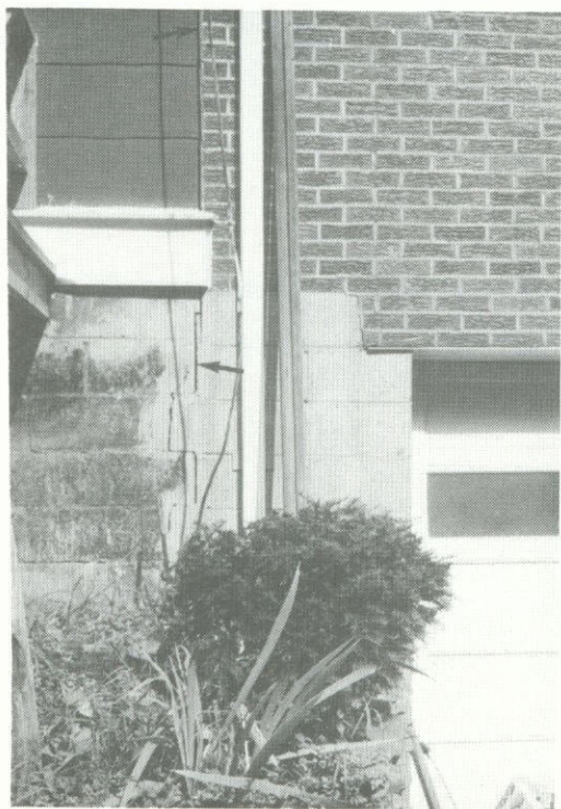
Fig. 4. Separation on the southeast wall. (after Peng and Hsiung, 1986)
