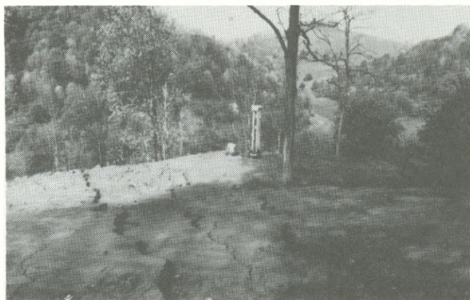
Fig. 14. Shows numerous tension cracks on the surface during monitoring of BH1.
