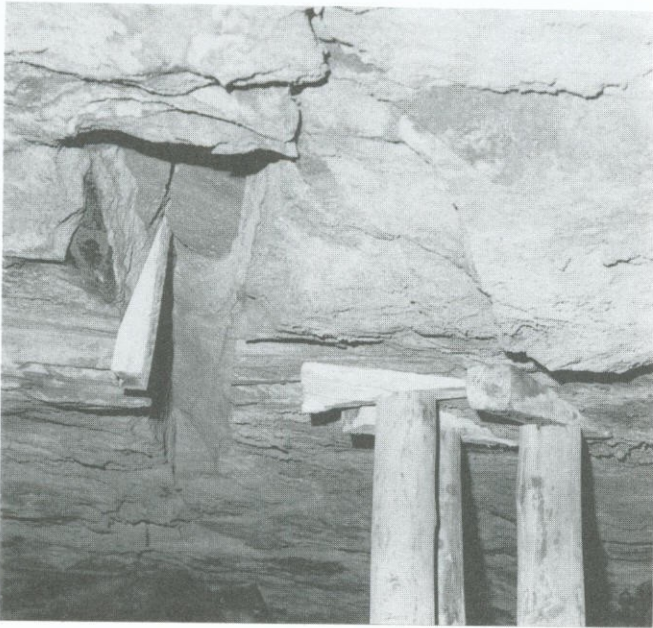
Figure 8 Warning wedges placed into the cracks.
