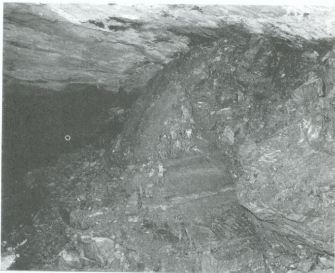
Figure 9 Illustration of the larger blocks into which the inner portions of the pillars had failed and the wavy nature of the roof.
