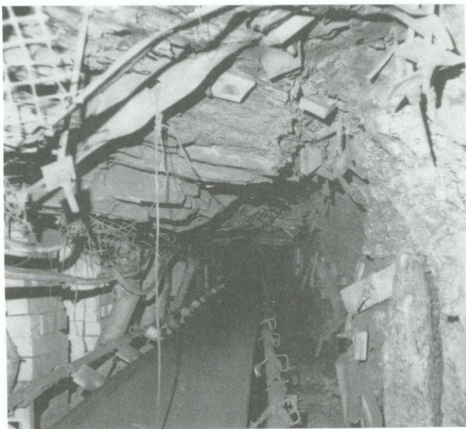
Figure 4. Cutter Roof Along Low Side Rib.
