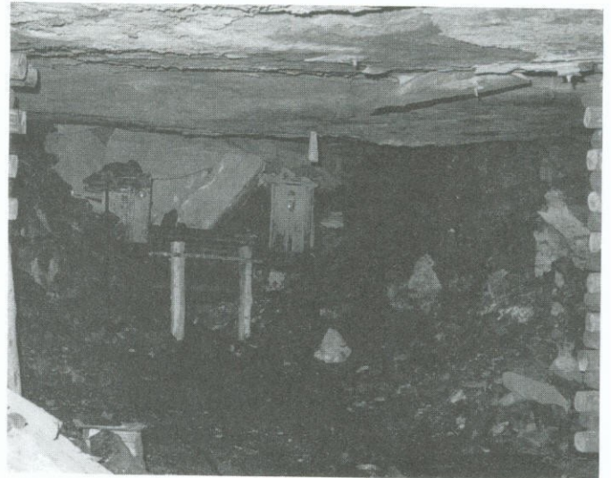
Figure 10 The shuttle car that was trapped by a roof fall, blocking the road to the other equipment.
