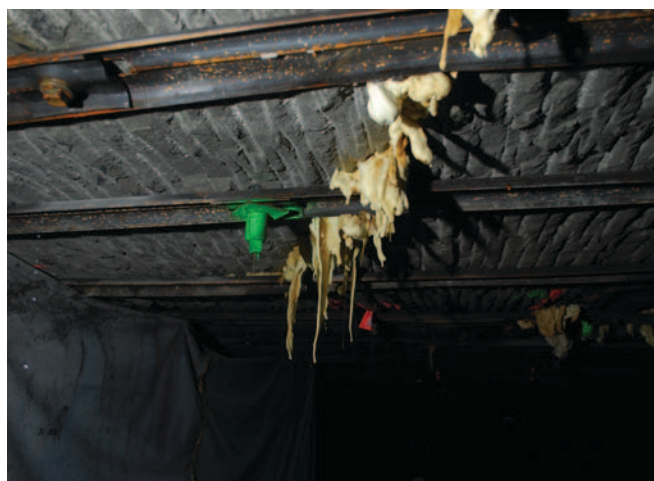
Figure 12. Polyurethane migration at roof line.
