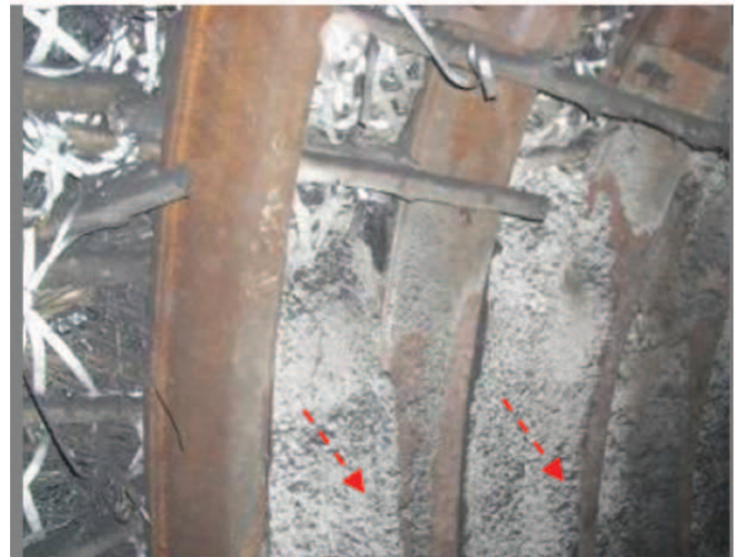
(b) Broken coal rib squeezed out into the gateroad
