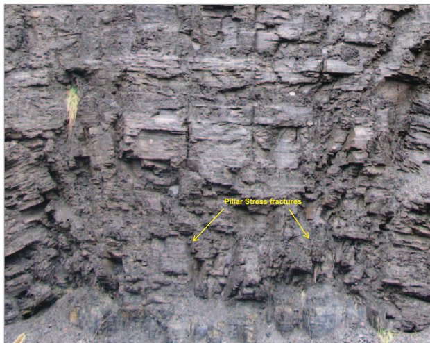
Figure 2. Stress relief fractures indicating the pillars in the process of yielding.
