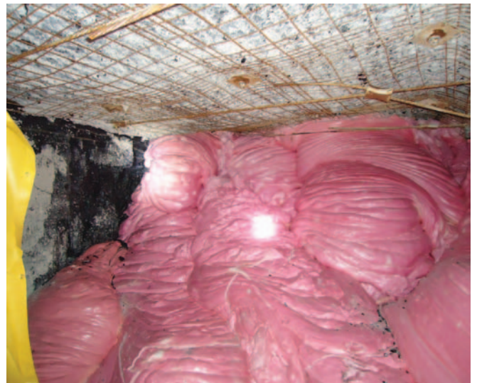
Figure 11. Phenolic foam underground.
