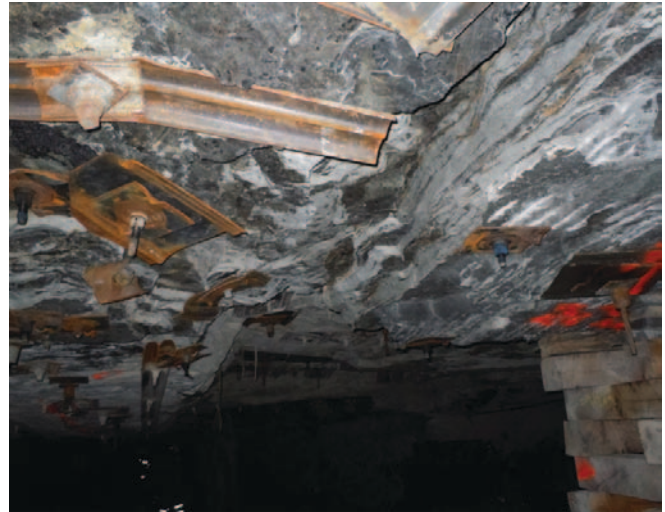
Figure 14. Signs of roof movement.
