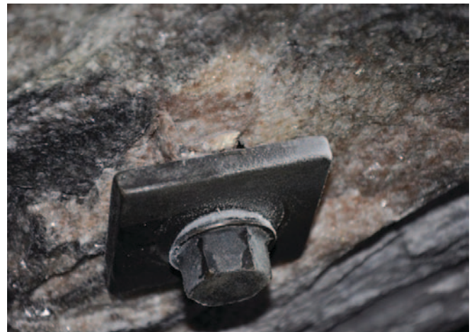
Figure 9. Installed Screw Anchor.
