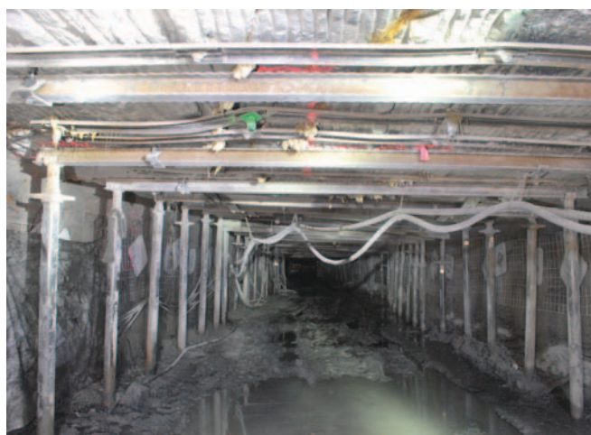
Figure 11. Polyurethane migration at roof line.
