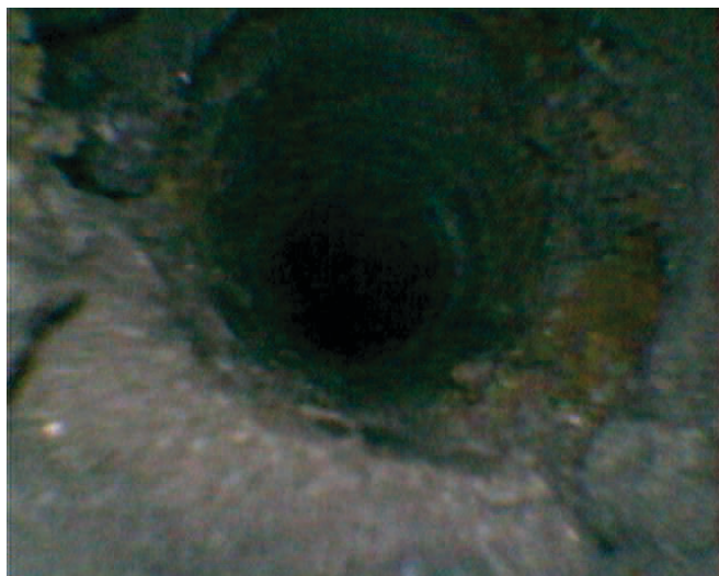
Figure 9. Roof weathering observed in test hole.
