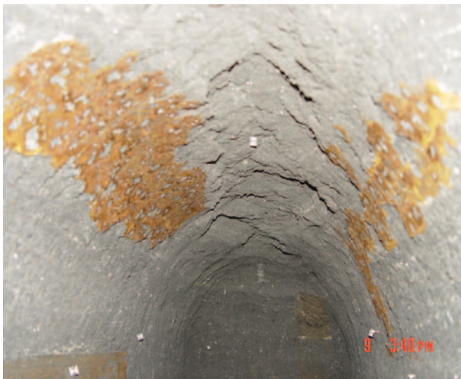
Figure 6. The roof of roadway damaged seriously.
