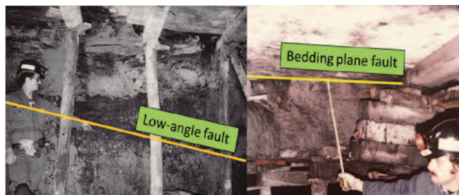
Figure 9. Photographs of faults observed within the Solar No. 7 mine. These faults are projected to intercept the Stoystown water supply wells.
