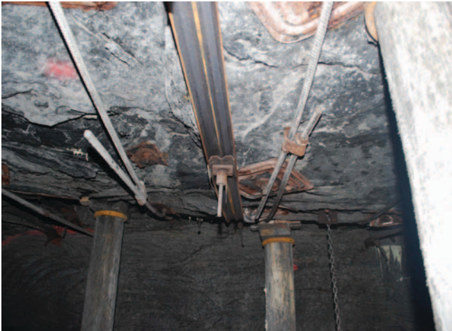
Figure 2. Channel forms to the roof line; truss cross-members leave unsupported gaps.
