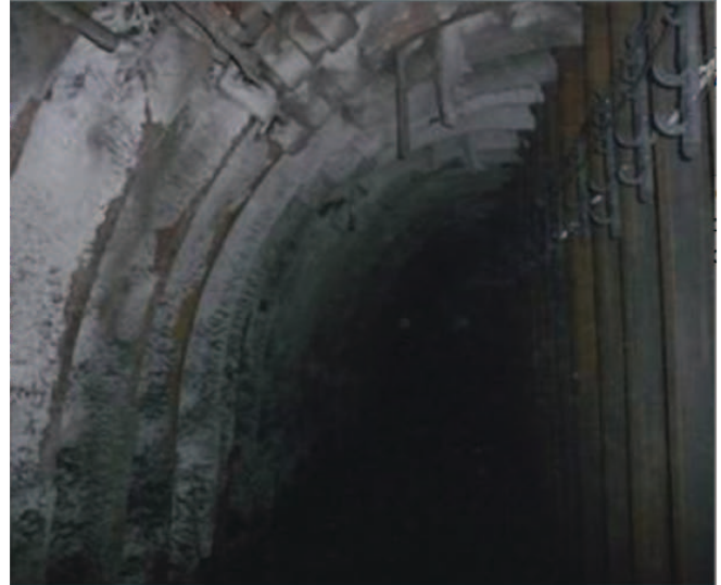
(a) Roadway deformation
