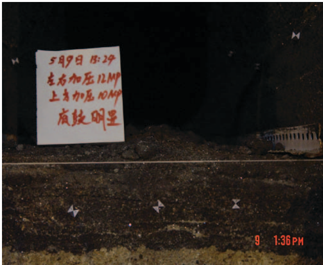
Figure 5. Floor heave of roadway.
